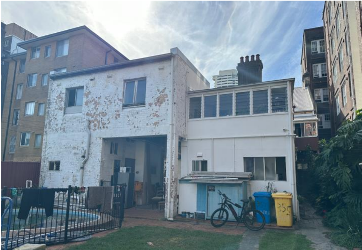
Figure 6: Rear setback of the subject site looking north towards rear of existing buildings on site
